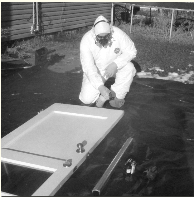
A SEICAA Weatherization crew member works on a door after replacing an existing door bottom to prevent air leaks.
